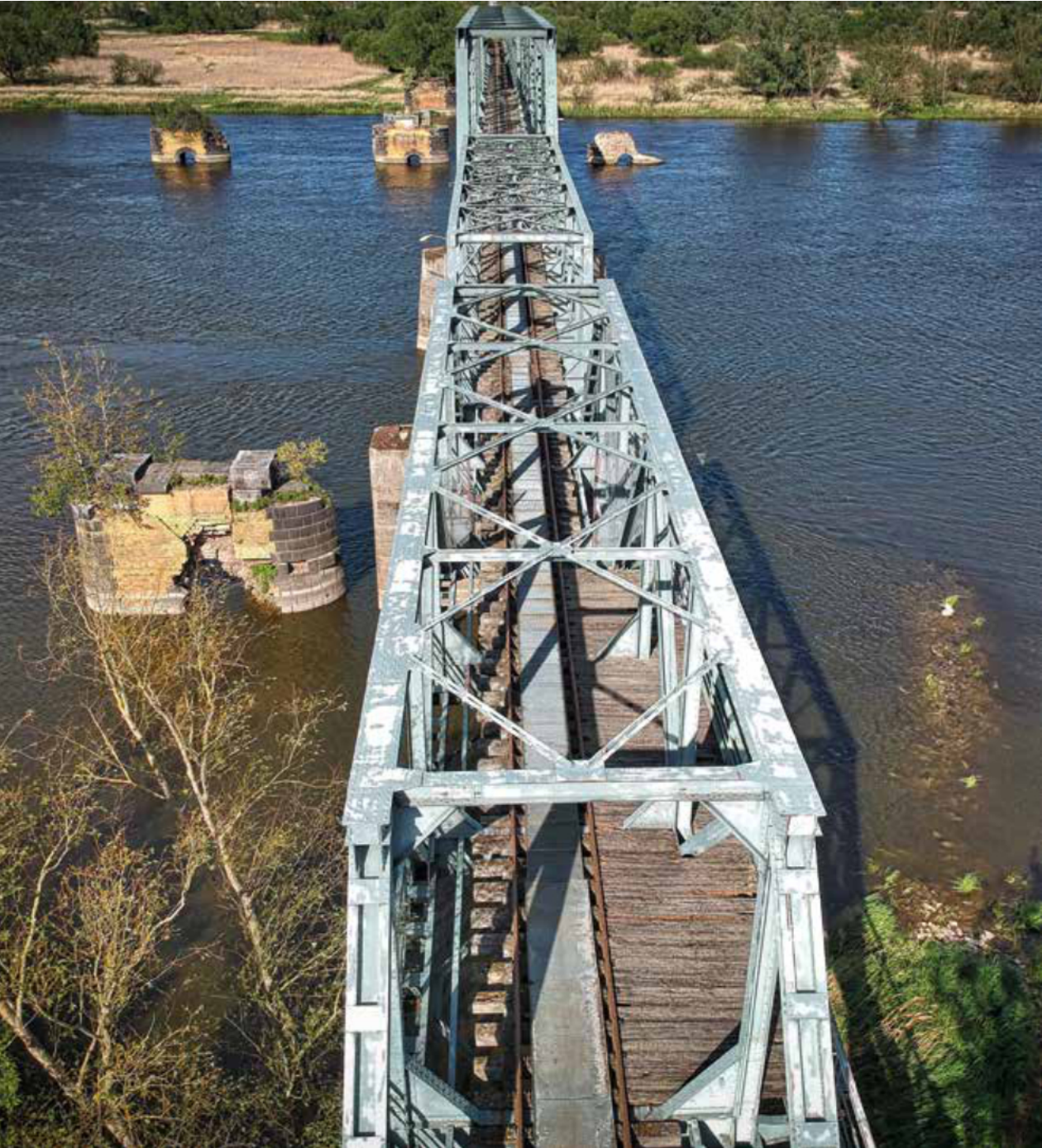
The Villages of Neurüdnitz (DE) and Siekierki (PL) are connected by a train bridge named »Europabrücke«. The restoration of this listed monument has started 2020 and will be finished for the use of travelers on foot and bike by 2022.
